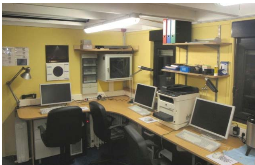
Computer and controll station of the entire facility
